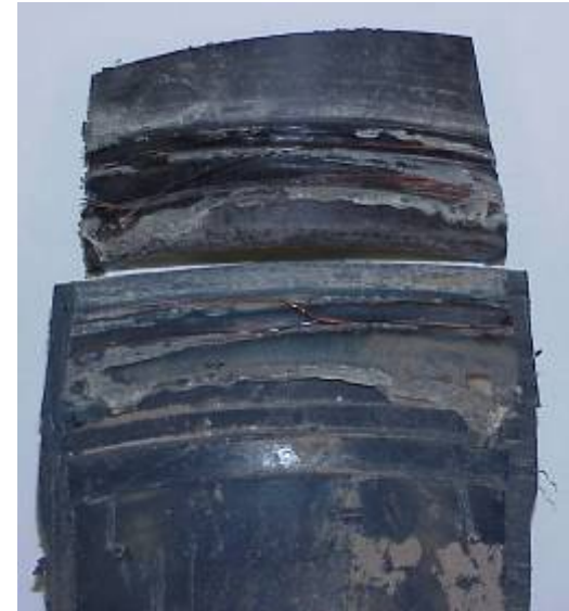
Pipe and fitting were not cleaned!
